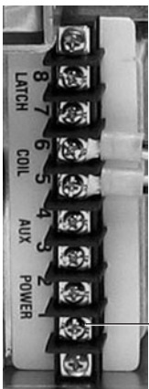
Control Terminal Strip
